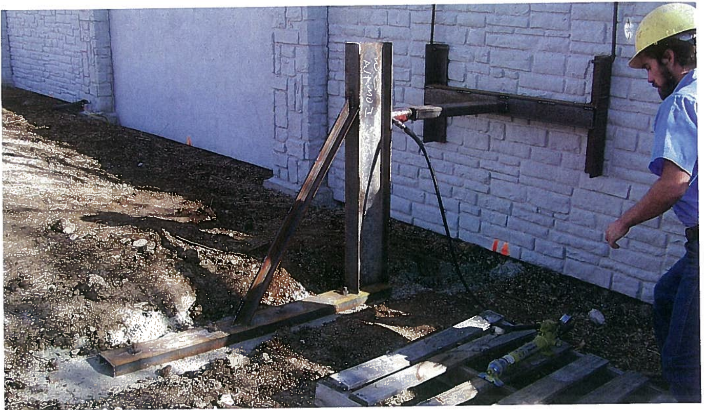
Tests were performed on a fence line that was installed with footings to demonstrate the behavior in the real world. The test results of walls reinforced with fiber and less steel were surprisingly impressive.
