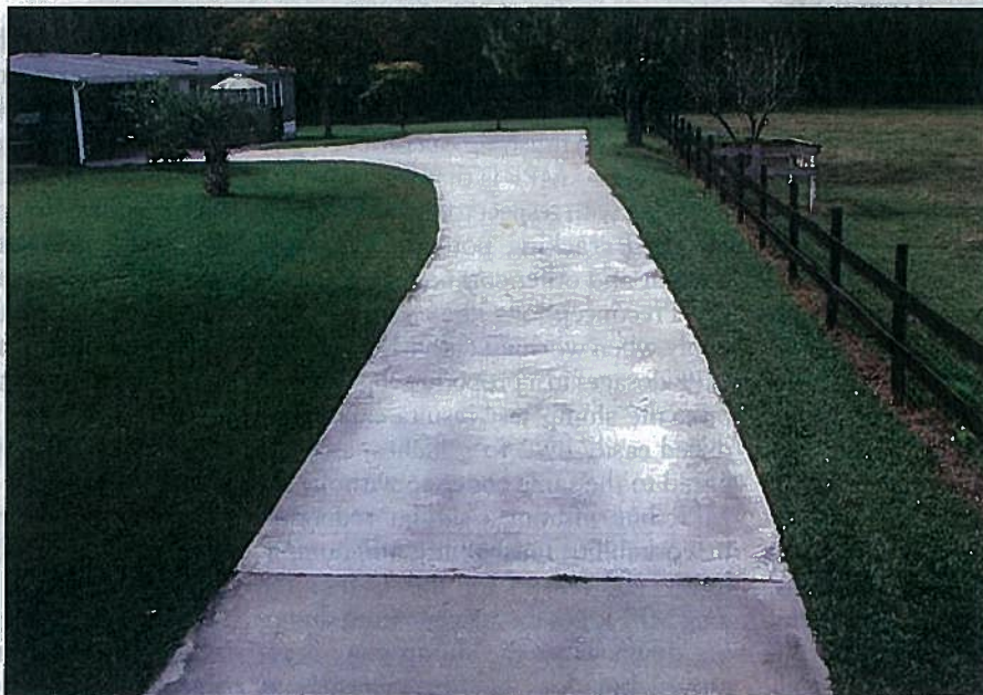
122x10-foot truck driveway flaring to a 43-foot-width with no joints and only one tight crack after four years. Photo: Alicia Simonelli
